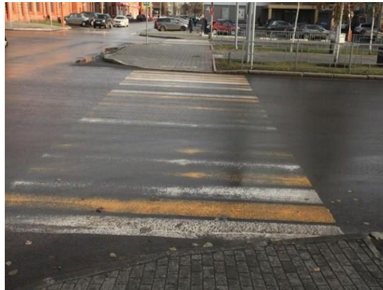
Figure 3. Road markings on the asphalt are washed off.
